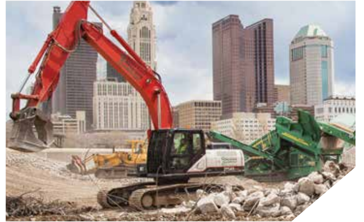
JDM Equipment used reprocessing equipment purchased with funding from the Clean Air Resource Center on the demolition of Veterans Memorial Auditorium in Columbus. The equipment crushes large pieces of concrete into a reusable stone product.
